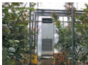
Air-conditioning equipment for a greenhouse
