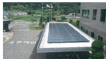
Photovoltaic power generation system (on the carport roof)
