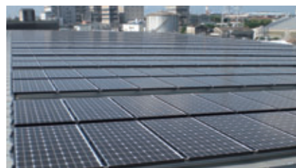
Photovoltaic power generation system (on the roof of the plant building)
