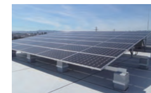
Photovoltaic power generation system (on the roof of the plant building)
