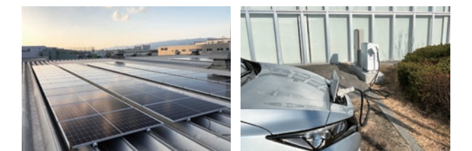
50kW of solar panels installed on the factory roof
